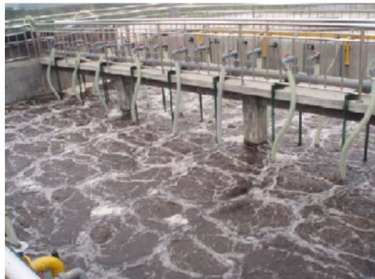
Figure 3. Submerged Membrane Bioreactor
